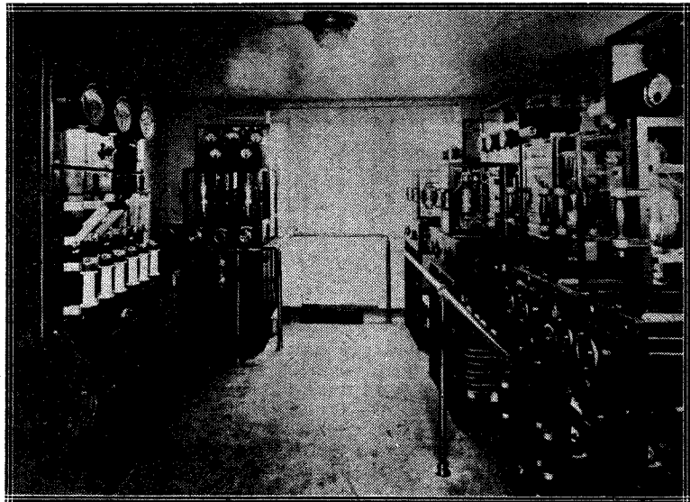
At the Brussels broadcasting station a Marconi 6kw. transmitter is used. The rectifier panel may be seen on the left, while on the right are the independent drive, main oscillator and modulator panels.
