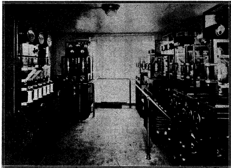
At the Brussels broadcasting station a Marconi 6kw. transmitter is used. The rectifier panel may be seen on the left, while on the right are the independent drive, main oscillator and modulator panels.
