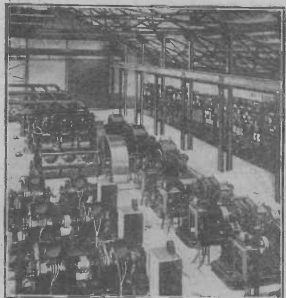
Generators and switchboards at the new G.P.O. beam station at Bodmin, Cornwall.
