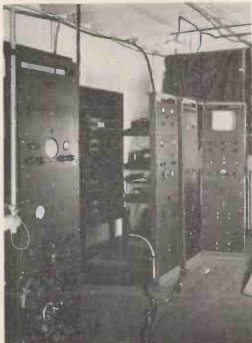
The racks containing the scan generators line amplifiers, synchronising generators and monitor tubes.
