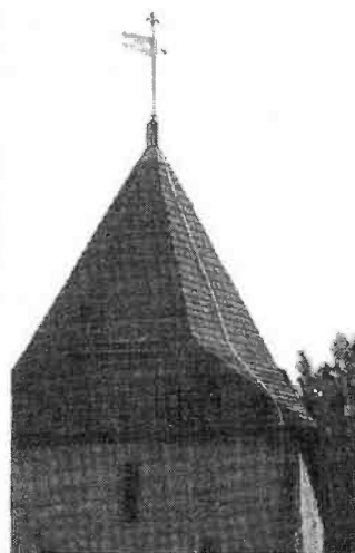
Fig. 1: Lightning arrester on church spire.
