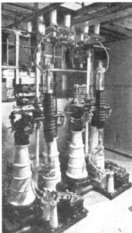
The final stage of the modulator unit in the Empire Station at Daventry. The mechanical water interlocks, which prevent the supply of power to the valves until the cooling water is flowing, are clearly visible.
