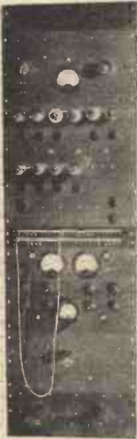
The transmitter control panel.
