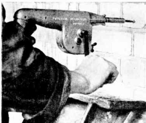
Fig. 4. —A MECHANICAL HAMMER BEING USED TO DRILL A HOLE IN A BRICK WALL.
