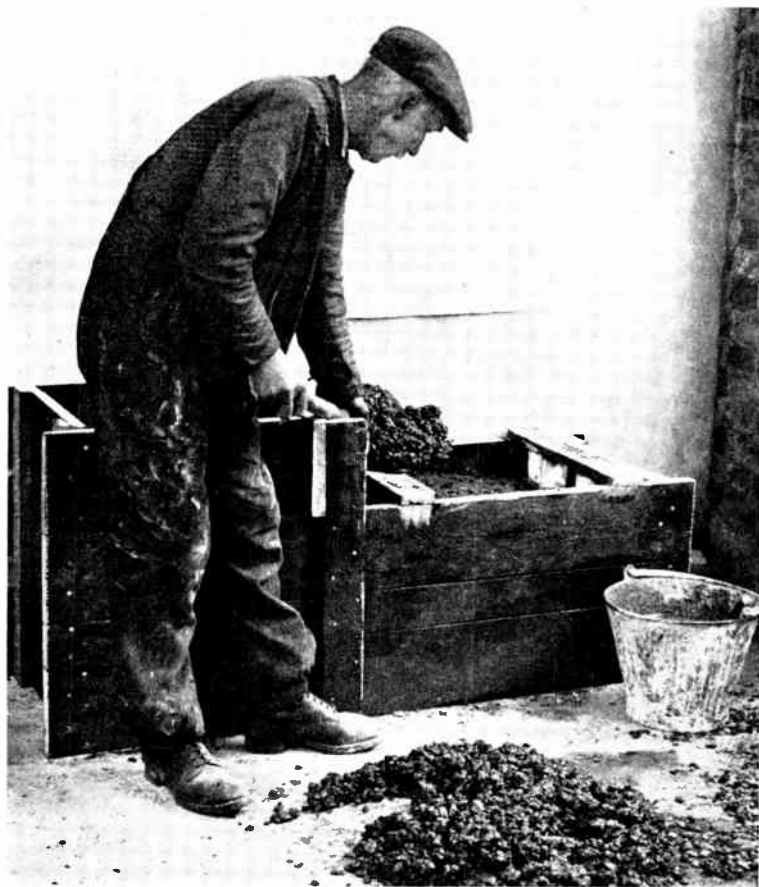
Fig. 1.—MAKING THE CONCRETE BED FOR AN ELECTRIC LIGHTING PLANT. (Stuart Turner, Ltd.)
