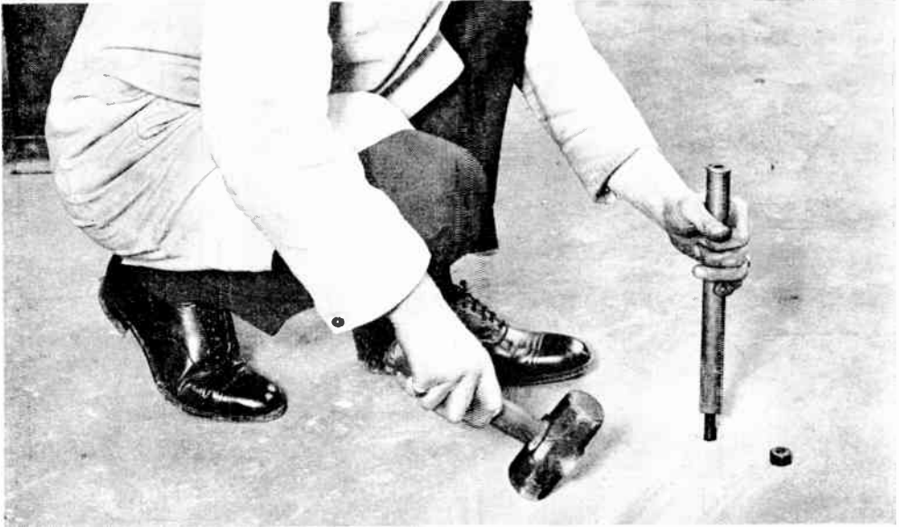
Fig. 13. —How to Fix Heavy Machinery to a Concrete Floor (3). The caulking tool is placed over the bolt and the caulking then carried out with a heavy hammer.
