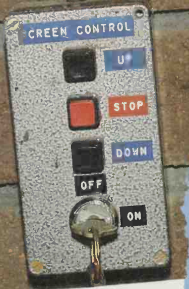
Photo 6. Automatic projector screen control panel.
