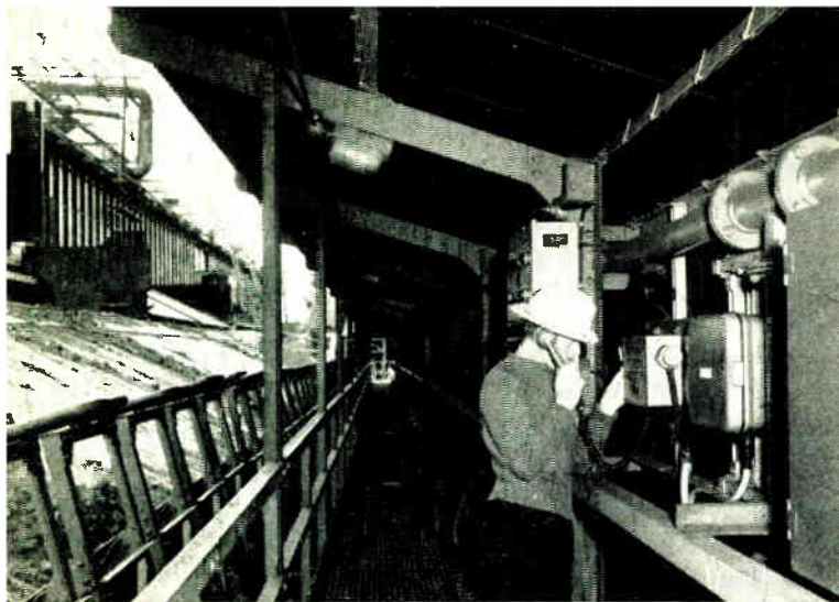
Shown is a 5-way A.E.I. telephone unit in the coke wharf section of the plant
