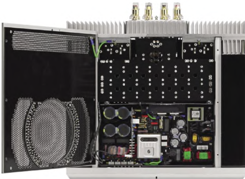
The top view shows the switch-mode power supply, with its many transformers and capacitors, is situated at front. Although switch-modes have transformers, they are not big and weighty like traditional types, because the conversion process works at high frequency.
