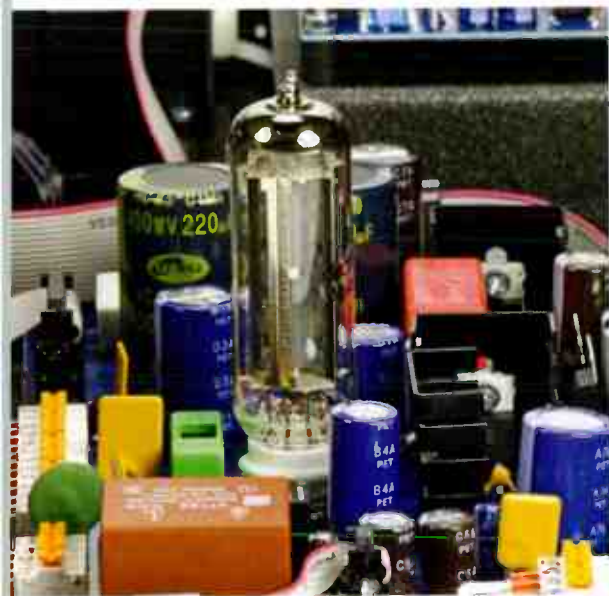
The 6CA4-EH valve (equivalent to an EZ81) acts as rectifier for the incoming mains.
