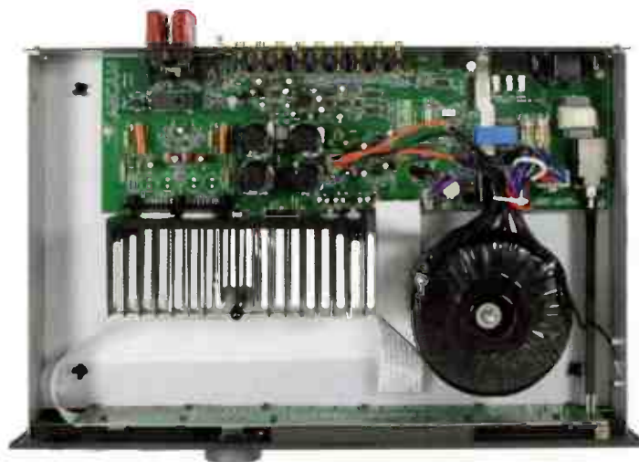
A hefty toroidal transformer dominates the interior
