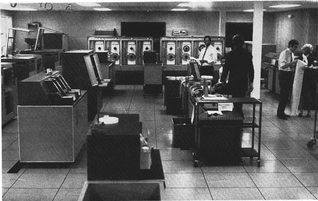
Fig. 4 General view of the computer room showing the control consoles (right), card readers (left), and tape decks in the background
