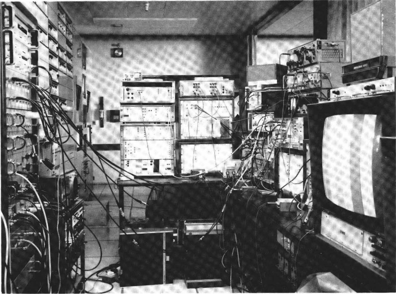
Fig. 4 60 Mbit/s digital video and audio satellite-transmission experimental equipment. The Post Office four-phase modulator and demodulator is on the left. The BBC baseband equipment is at the centre and on the right.
