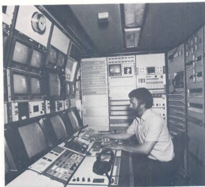
The Engineering and Camera Control Area
