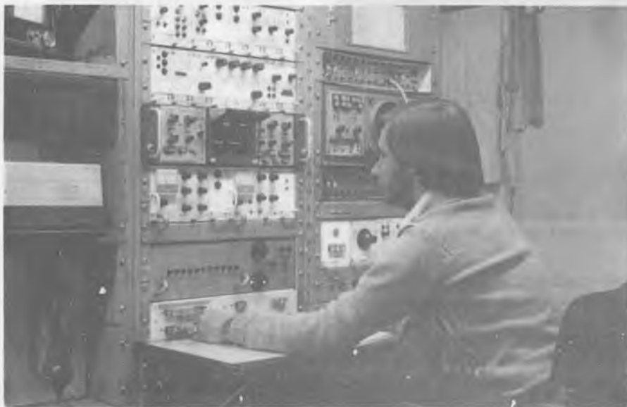
Keith Moore, shift engineer, measuring tv test signal parameters, in the Switching Centre
