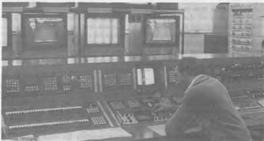
David Bonor, shift engineer, operating the Switching Centre central desk
