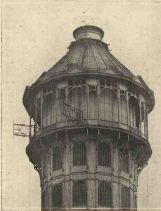
Fig. 1.—Sound and vision ultra-short-wave aerials on the Crystal Palace South Tower balcony with the new high-power U.S.W. vision aerial at the top of the tower.
