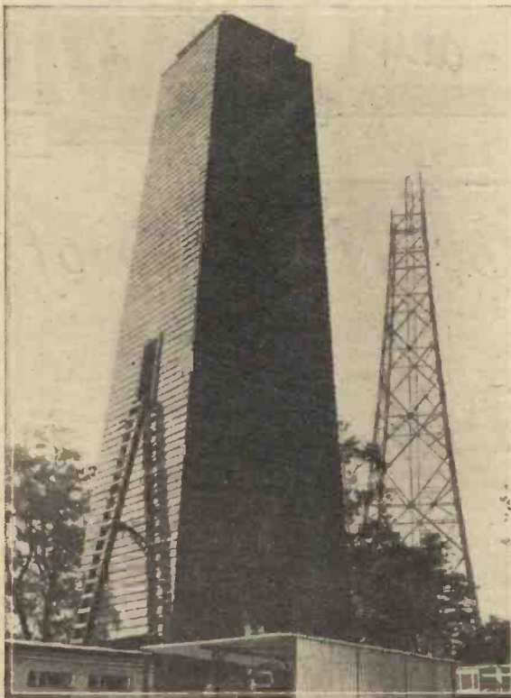
In connection with the new broadcasting station in the Forest of Tegel, the aerial masts are constructed entirely of wood with the aerial running vertically through the centre. In the illustration, a partly completed mast is shown, and in the foreground is a water tower for the valve-cooling apparatus.
