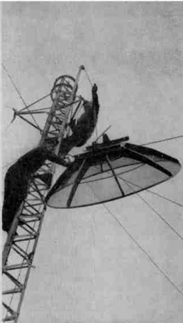
Corporal Guy Beaupre and Corporal Len Brandstad (top) hoist into position the disc-shaped antenna which transmits and receives messages.
