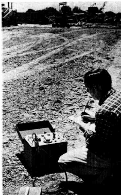
Operator obtains final surface density (or surface moisture) reading on the construction site. The scaler has counted impulses received from the surface probe — the total count appearing on the scaler's five glow tubes. The "count" is applied to a factory supplied calibration chart for a direct density reading.
