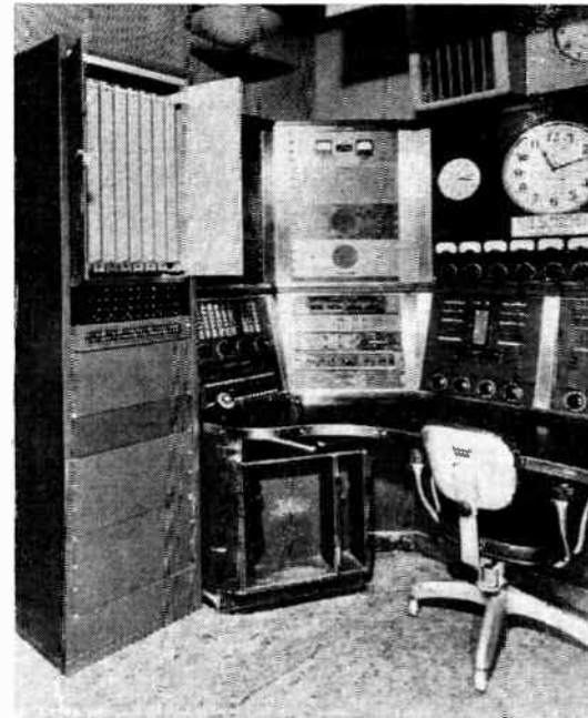
● STUDICON—MASTER CONTROL SECTION (shown at left with doors open), located in the master control room of Radio Station WOR, New York City. The master control section is the electro-mechanical heart of the Radio Studio Control Switching System.
