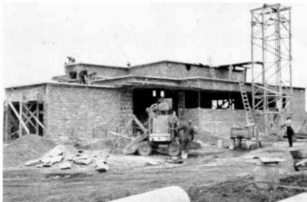
Terra Cotta tile was completed at Lacombe in October. Steel windows have since been installed.
