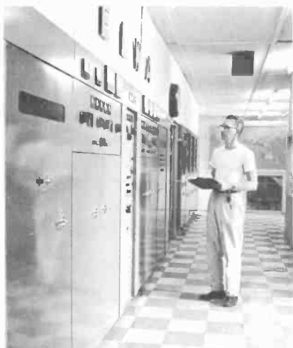
Technician Dave Naff reads the meters on 50 kw transmitter.
