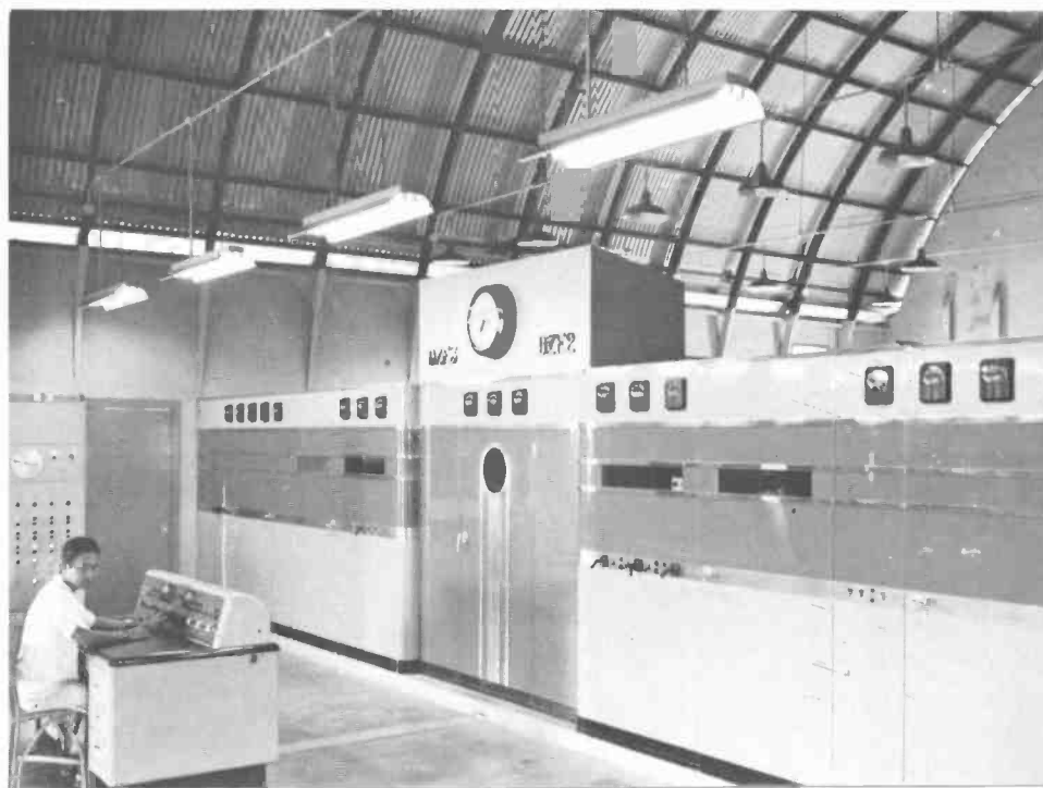
50,000-watt RCA overseas transmitter. Chief engineer, Francisco Matias, at controls, Bocaue, Philippines.
