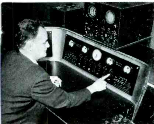
Master control board of NBC's television transmitter station, located on the 85th floor of the Empire State Building.
