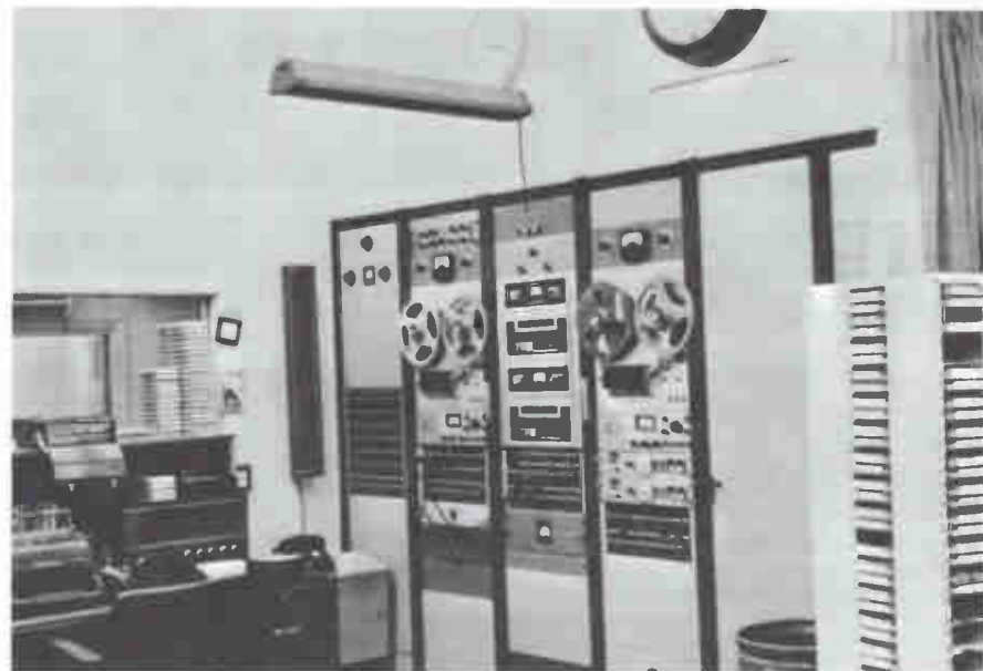
Fig. 16-15. Washington line recording racks in KYW's news gathering facilities.
