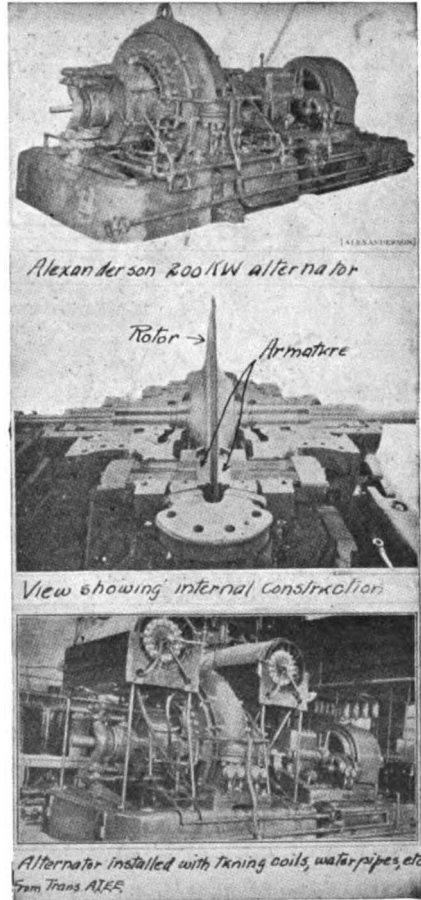
FIG. 17. Views of the high-powered Alexanderson generator installed at New Brunswick; over the alternator (in the lower view) may be seen the oscillation transformers which connect the generator to the antenna.
