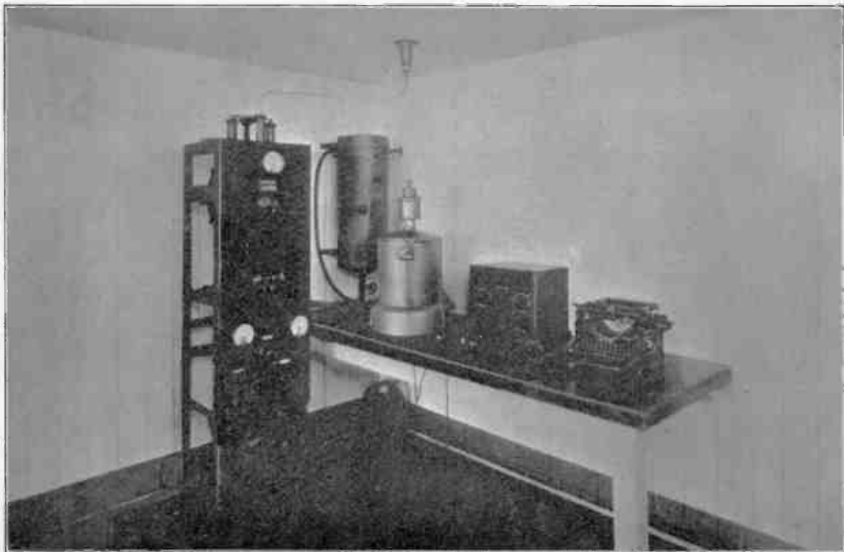
PLATE I.—Two-kilowatts Federal arc installation. (Courtesy, Federal Telegraph Company.)
