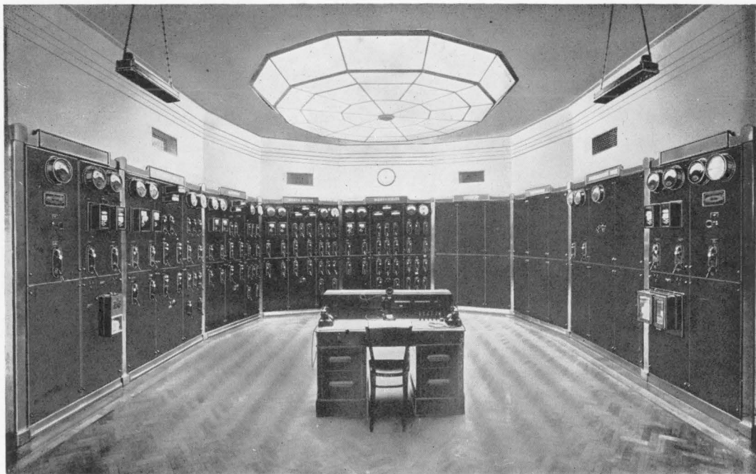
FIG. 48.—A view of a remote control switch and instrument board for a steel tank rectifier sub-station. (G. E. C.).
