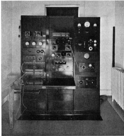
FIGURE 28. A General Radio frequency monitor installed at station WCSH, Portland, Maine. The monitor is shown at the top of the right-hand bay
