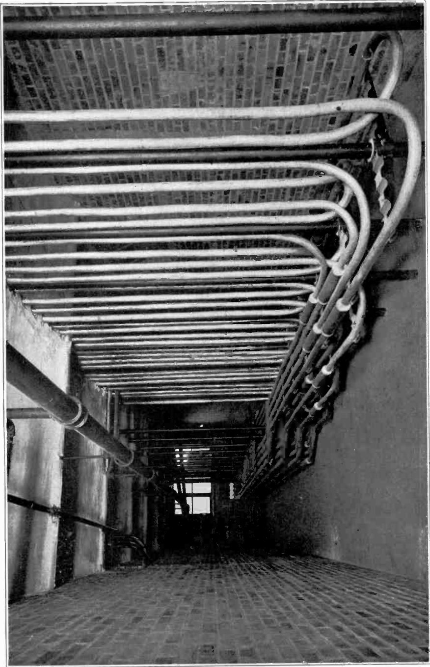
CABLE ENTRANCE TO LARGE TELEPHONE OFFICE BUILDINGS The Cables Enter the Basement from the Street Ducts and Pass in a Single Row through a Fireproof Floor Directly to the Distributing Frame Above.
