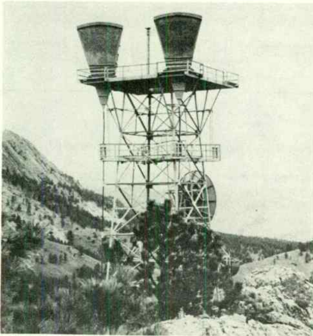
Figure 5-11. A Repeater Station. (Courtesy of Southwestern Bell Telephone Co.)
