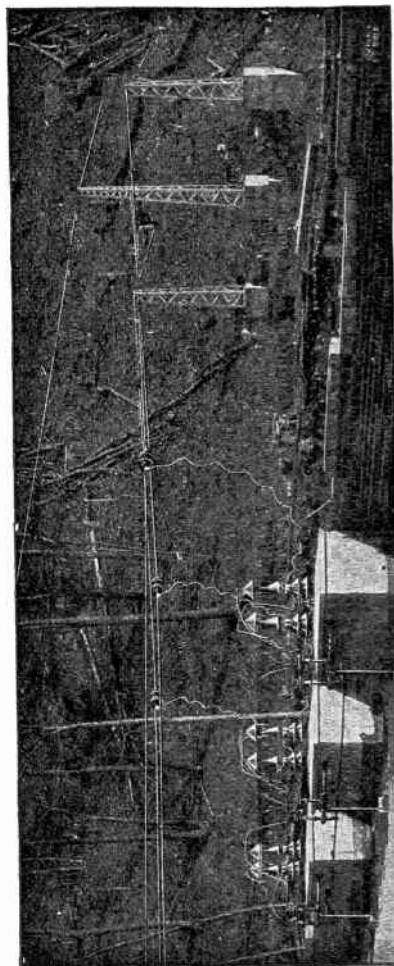
FIG. 2,174.—View from roof of power house of the Schaghticoke-Schenectady transmission line, showing anchor poles, strain insulators, lightning arrester horn gap and line entrance bushings.
