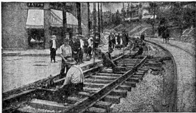
FIG. 7,925.—Chicago "Little Giant" electric track-drills reaming joint holes on the tracks of the Pittsburgh Railways Co.
