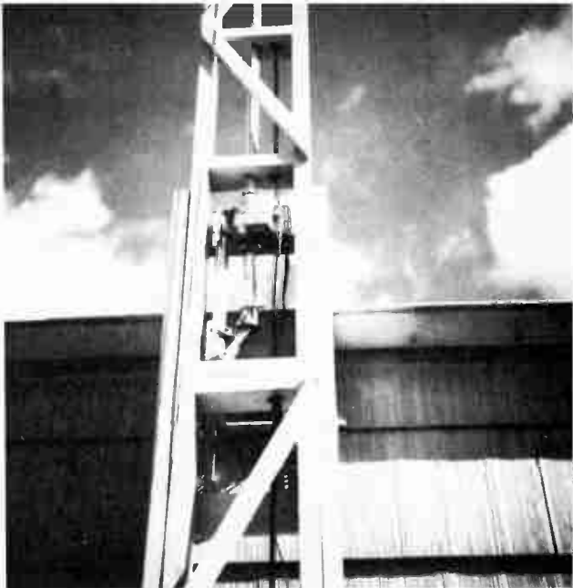
Fig. 21-59 — This close-up shows the rotor and cable installations. A double 2 X 4 is used as the base support for the rotor.
