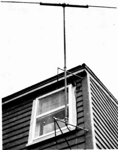
Fig. 14-61—Over-all view of the antenna and mounting. The feedline comes out of the bottom of the mast and through the wall into the shack.
