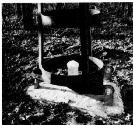
Fig. 60 — Hinged base of the N5BQA tower.
