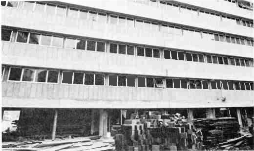
b. Headquarters (under construction) of TV Globo, a Brazilian television network. (Courtesy Rede Globo, Rio de Janeiro)
