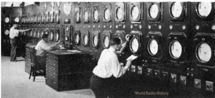
Above: Master control desk, nerve center of broadcasting in the RCA Building, designed and built by RCA Engineers. Left: Control board of the studio air conditioning plant.
