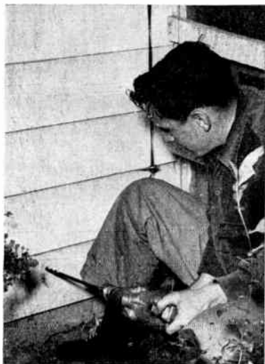
Fig. 10. Drilling a hole through the wall of a house into the basement for bringing in the television transmission line. (RCA Victor photo)
