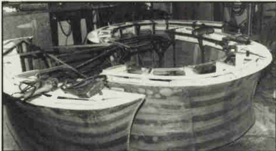
"Hourglass desks" in progress. The Luaan plywood stripping can be seen with the fiberglass coat applied. The light colored bands are 2" wide masking tape used to bridge the seams between the strips.
