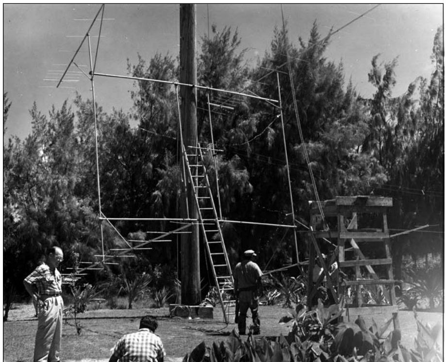
This picture shows Tommy (on the left) monitoring a crew of men ready to hoist the 56 element beam to the top of a 90’ utility pole. The others in the picture are “riggers” from RCAC.
