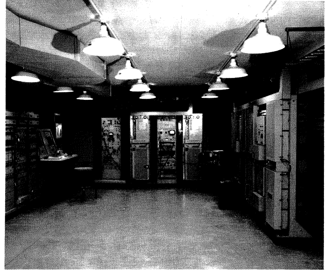
Figure 9. AN/FRC-39A(V) Quadruple Diversity Exciter, Receiver, Multiplex and Technical Equipment (low-level) Terminal.
