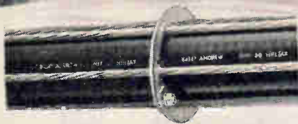
870-foot self-supporting catenary installation of 5-inch HELIAX air dielectric coaxial cable (Type HJ9-50) at mountain top site of Station KBYU-TV, Provo, Utah.
