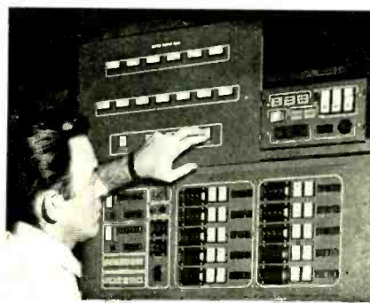
Whittaker control unit consists of monitor panel, top left, master control panel, right, and decoder box at bottom.
