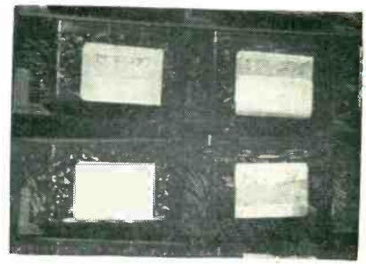
Closeup of wire-storing boxes
