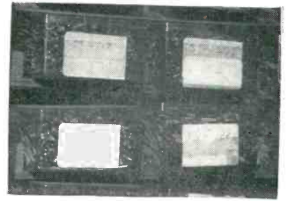
Closeup of wire-storing boxes
