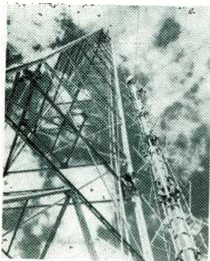
Super turnstile antenna for KECA-TV takes its place among the clouds atop Mount Wilson 6,000 feet above Southern California
