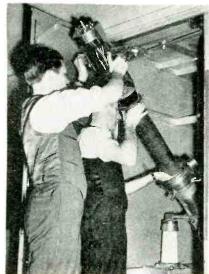
Two engineers install one of the 100-kw water-cooled transmitting tubes at the Government-owned short-wave station in Canada. A special beam antenna gives a total effective power of 10 million watts to the station
