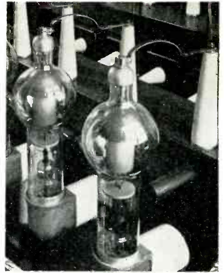
Cooling of high power rectifier tubes is provided by an air blast through the pipe behind each tube. This maintains the proper temperature for condensation of the mercury vapor in the tube
